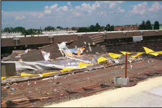
Safety barricades are installed around the areas of missing deck to ensure worker safety.
