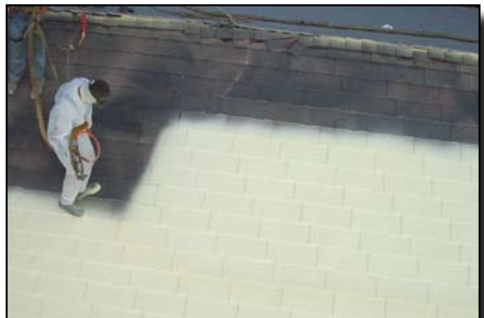
SPF over an asbestos shingle system.
