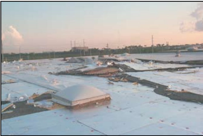
Twenty five thousand square feet of single ply roof membrane is completely blown off in the storm.
