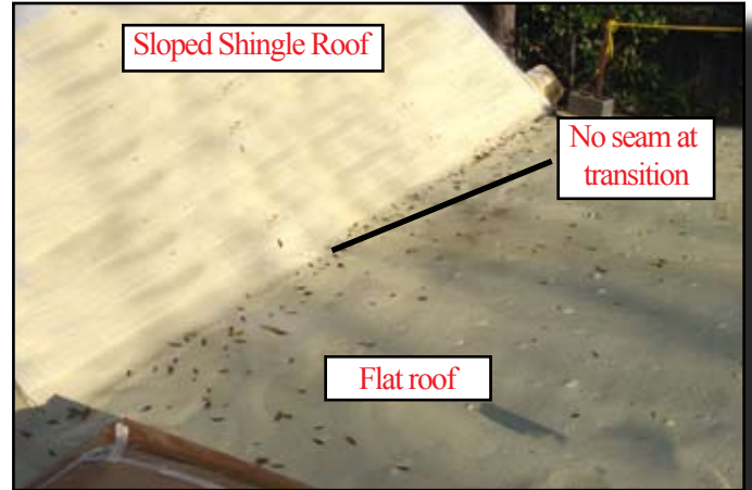
SPF over a sloped fiberglass shingle roof and flat deck. At the transition between the sloped and flat roof, the SPF is monolithic (one solid piece) with no seams to leak.
