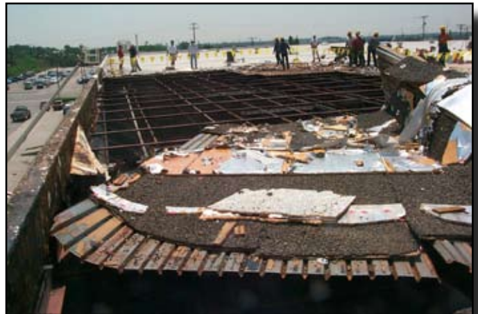
5,000 s.f. of metal deck is ripped from the structural purlins. Falling debris caused an unsafe condition inside the building.
