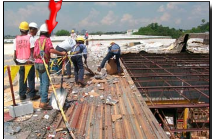
Crew members remove debris from the damaged area. Danger from falling debris was preventing entry into the structure.
