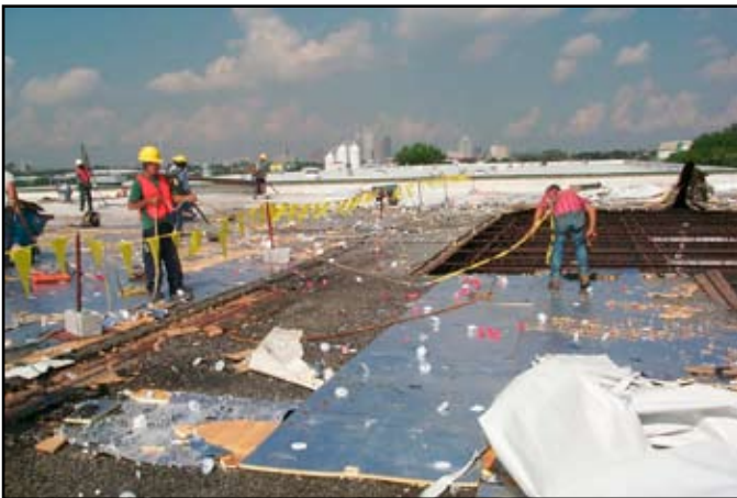
Fall protection is attached to all crew members that are working inside the safety barriers.
