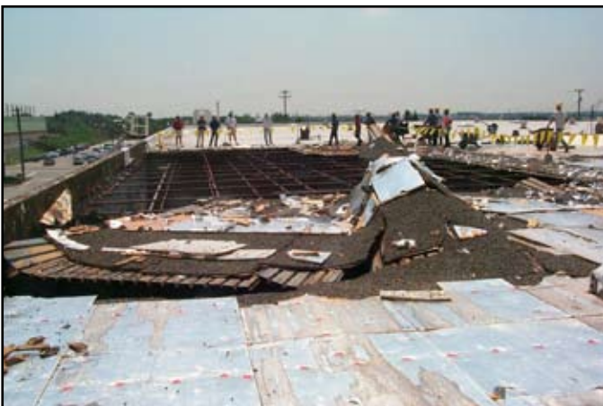
Metal deck is crumpled and lying in piles on the roof.
