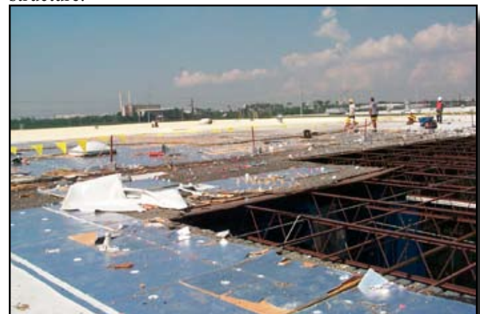
Area around the missing decking is secured and all debris is removed. Entry into the structure is now safe.
