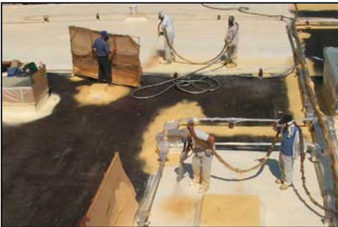
SPF over a modified bitumen.
