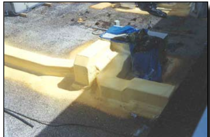
This duct work was crushed in many areas and water was pouring in the building. The entire duct was encapsulated with SPF.
