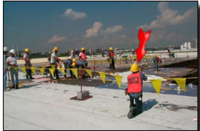
Four full time safety monitors are stationed around the perimeter of the area while crews work around the immediate area of missing deck.
