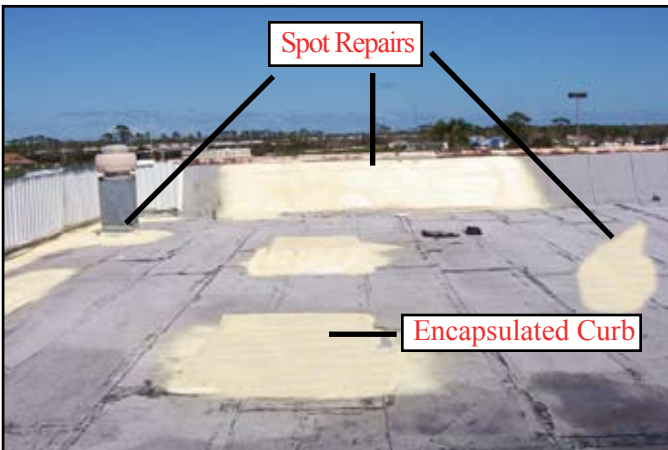
SPF used for spot repairs to a parapet wall and various areas on a modified bitumen. Note the curb that is completely encapsulated (the fan top had blown off.)
