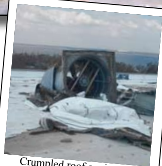
Crumpled roof equipment
