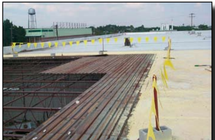
"Tie-in" area at the missing metal deck area (end of day one.)
