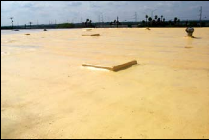
The finished SPF temporary roof system is seamless. No seams means no leaks.
