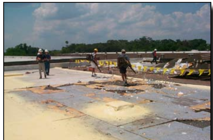
Loose debris is blown off the surface for better adhesion of the SPF.
