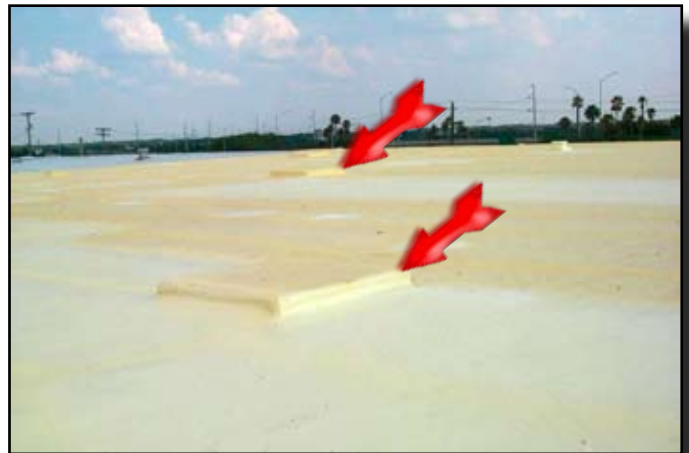
The A/C units were blown off these curbs. Installing plywood over the curbs then completely encapsulating them with SPF easily repairs this condition.
