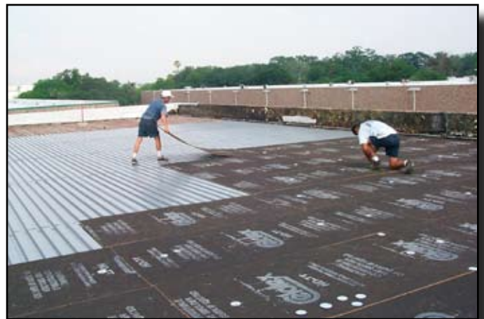
The insulation is attached to the metal deck with screws and uplift plates.
