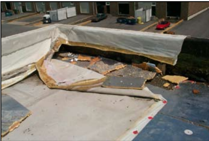
Missing wall flashing.
