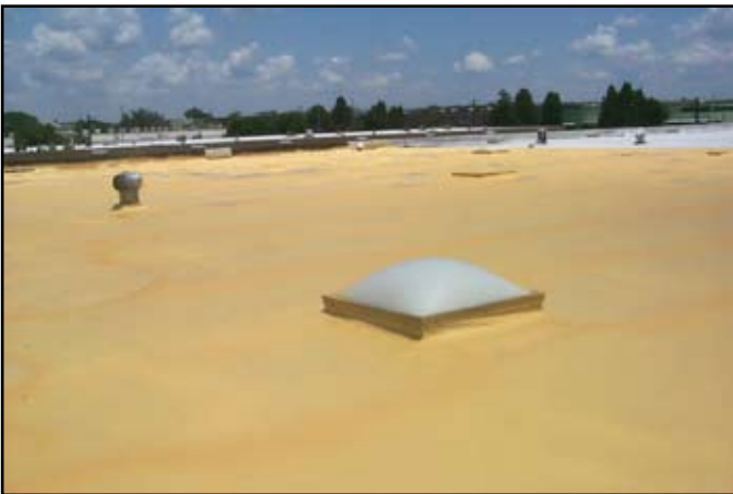
SPF is spray applied, filling all cracks and crevices. Skylights and other roof penetrations are easily sealed.
