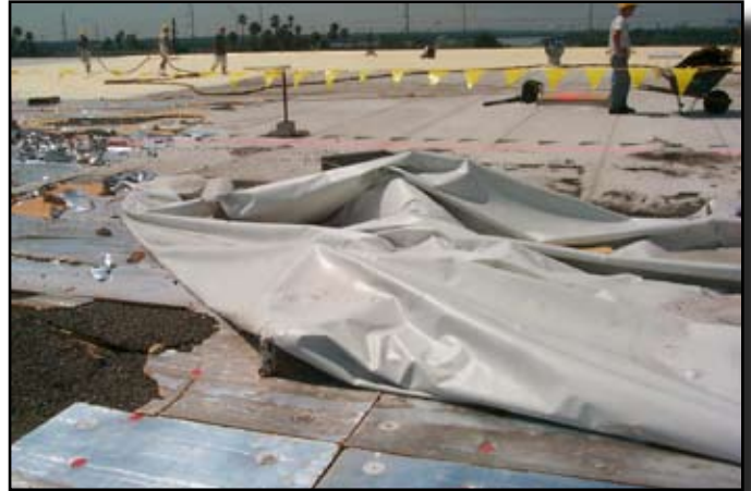
Torn and ripped single ply roof membrane.
