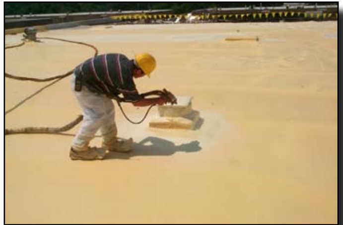
Curbs, skylights and wall transitions are quickly and permanently sealed with spray applied SPF.
