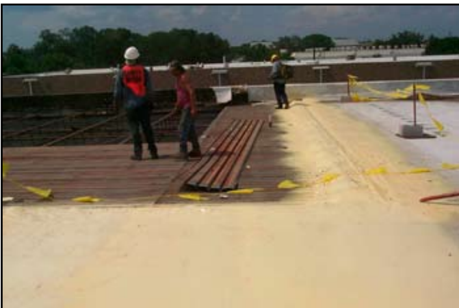
"Tie-in" area at the missing metal deck area (end of day one.)
